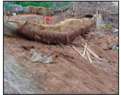
The soil-specific Silt Stop is then applied on top of the matting; the powder reacts with the metals and clays within the soil to bind it together. A series of wattles are placed in conjunction with the soft armoring and perpendicular to the flow to create a series of checks that will trap sediment and collect particulate created by a stormwater treatment system placed upstream.
