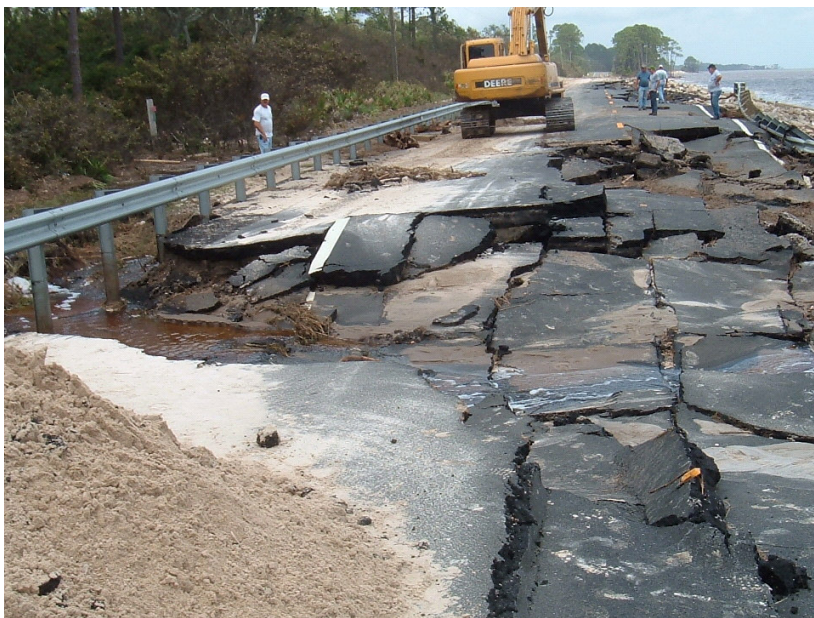
The movement of the highly erosive beach sands caused the roadway to collapse, in some places across the entire width of the two lane road.
