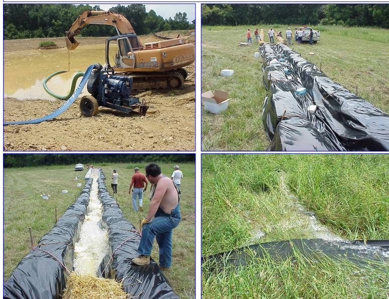
Top Left: Pond water having initial NTU of 700. Top Right: Site specific Floc Logs® secured in upper portion of treatment ditch. Bottom Left: Pond water being pumped into treatment ditch. Bottom Right: Water flowing off-site having NTU of 2.1.
