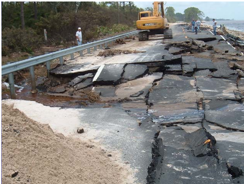
The movement of the highly erosive beach sands caused the roadway to collapse, in some places across the entire width of the two lane road.
