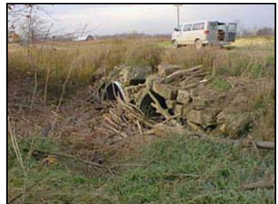
Debris and sediment choked crossing
