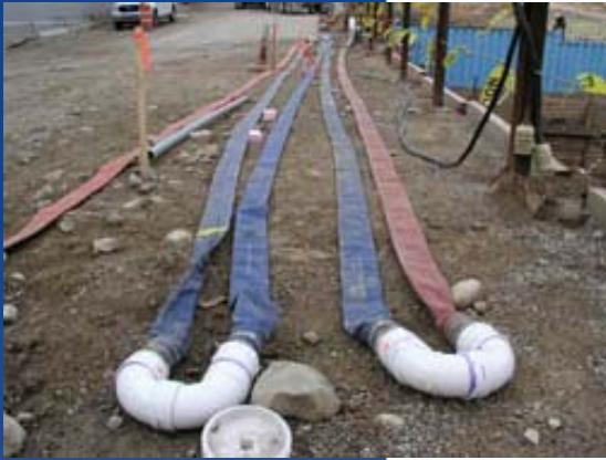
Hard-pipe turns used to conserve space
