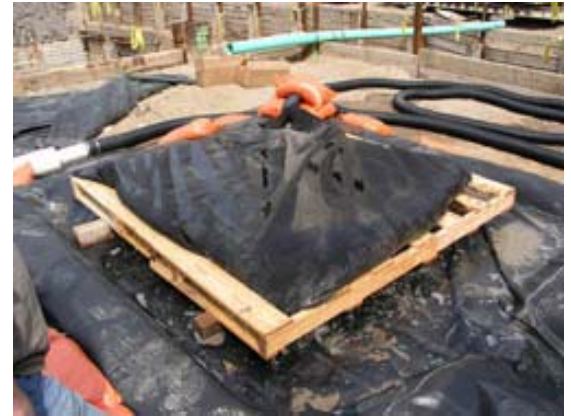
Background: 2nd wye element discharge into plastic pipe Foreground: Filter bag collection of floc and chelates
