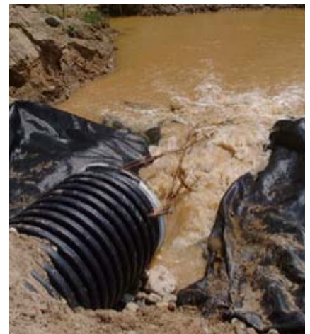
Grit pond effluent with attached Floc Logs ®
